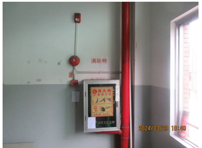
Fire hydrant and alarm
