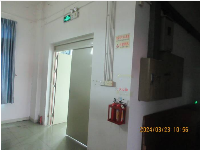
Emergency exit marked with exit sign and emergency light
